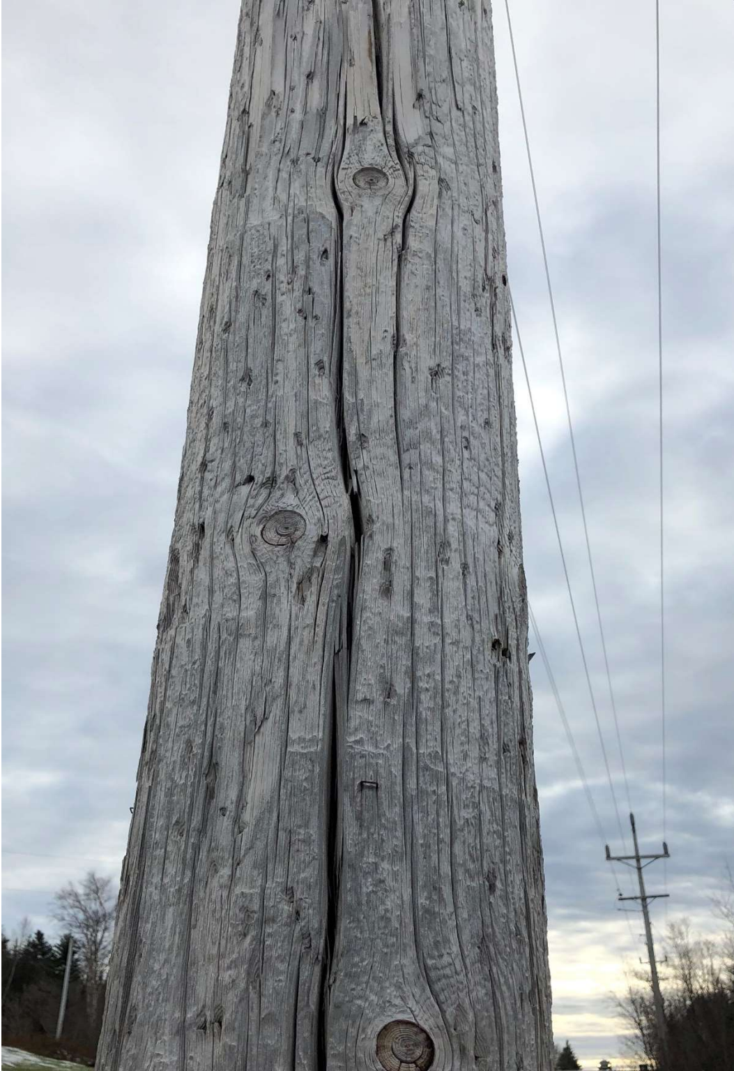
Figure A-1: Deep Splits Through Hollow Pole
