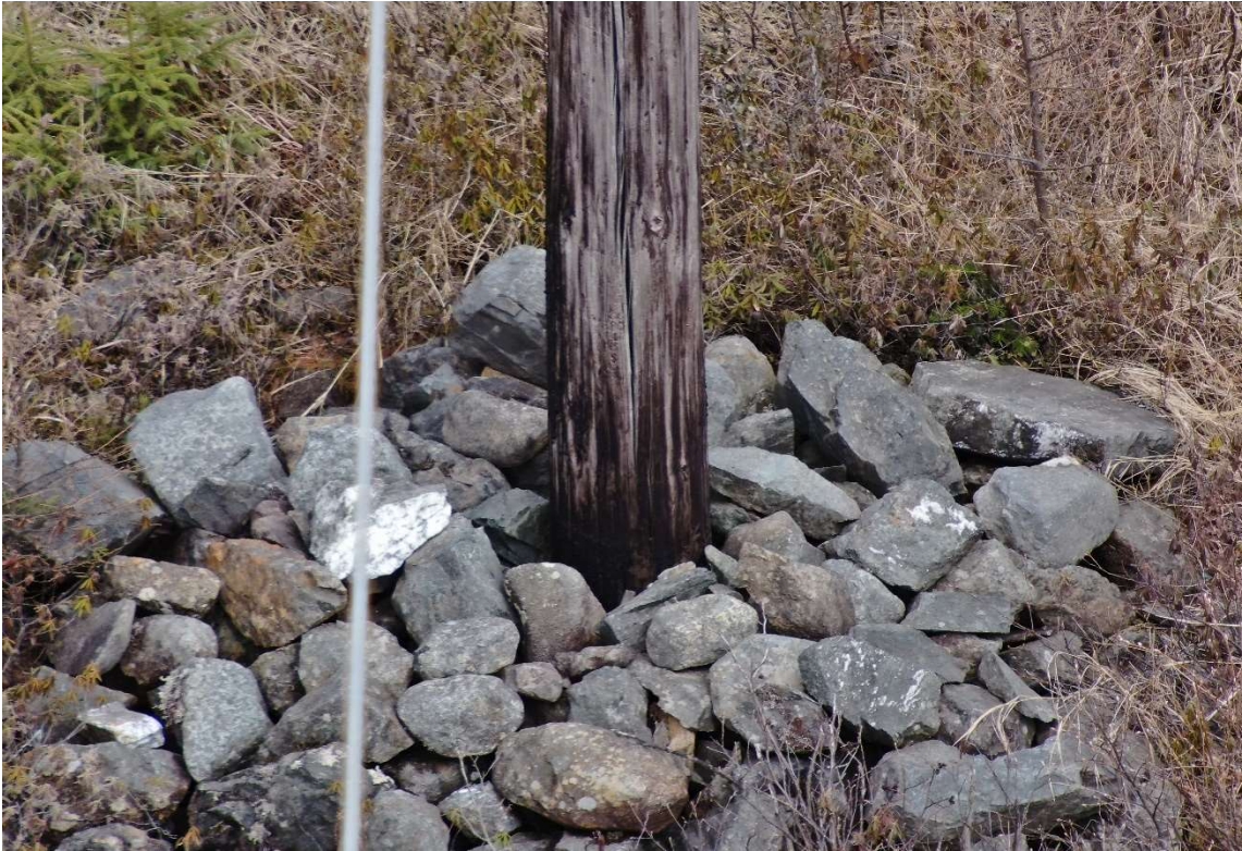
Figure A-9: Missing Timber Crib and Splits in Pole
