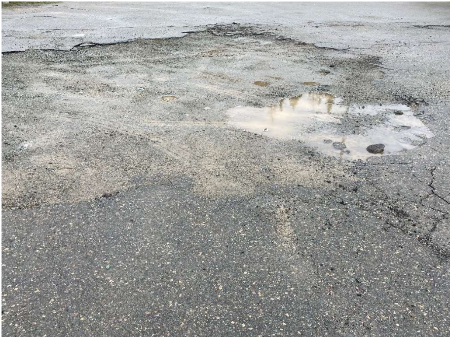
Figure 9: Deteriorated Asphalt Parking Lot
