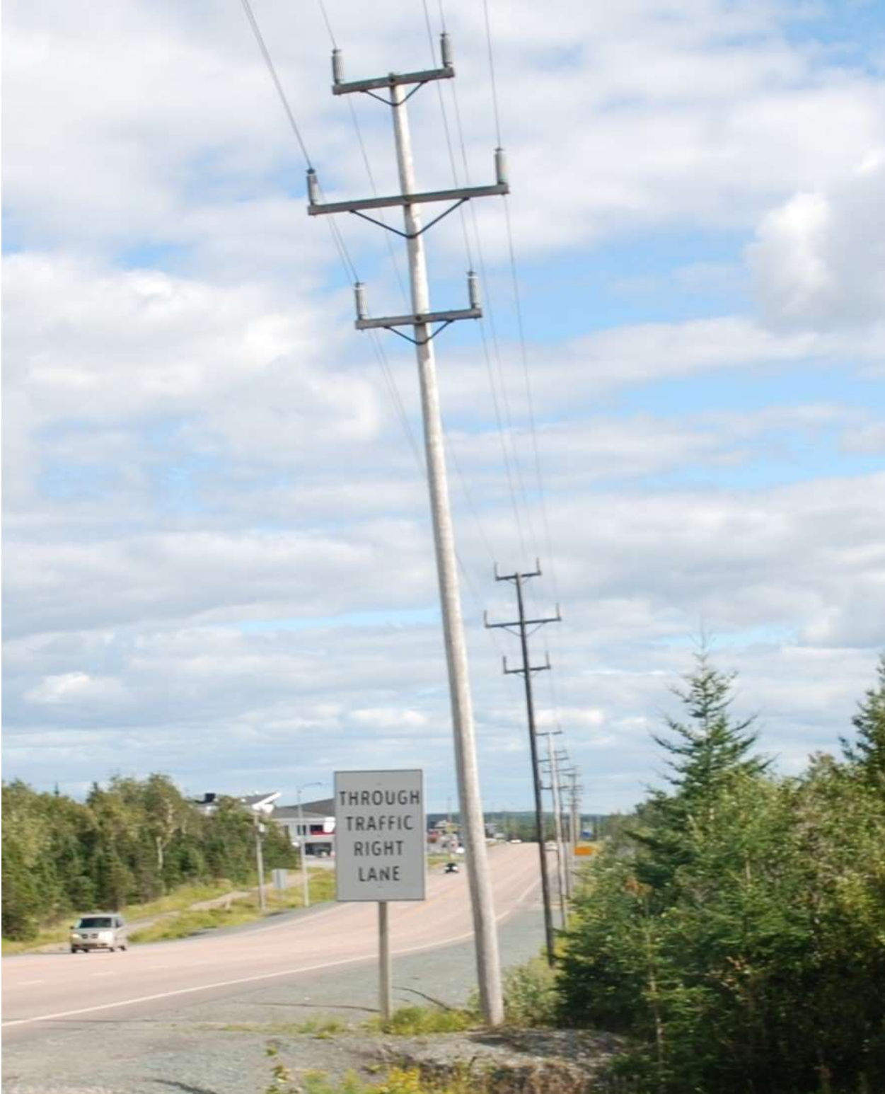
Figure A-10: Leaning Structure (Double Circuit Structure)
