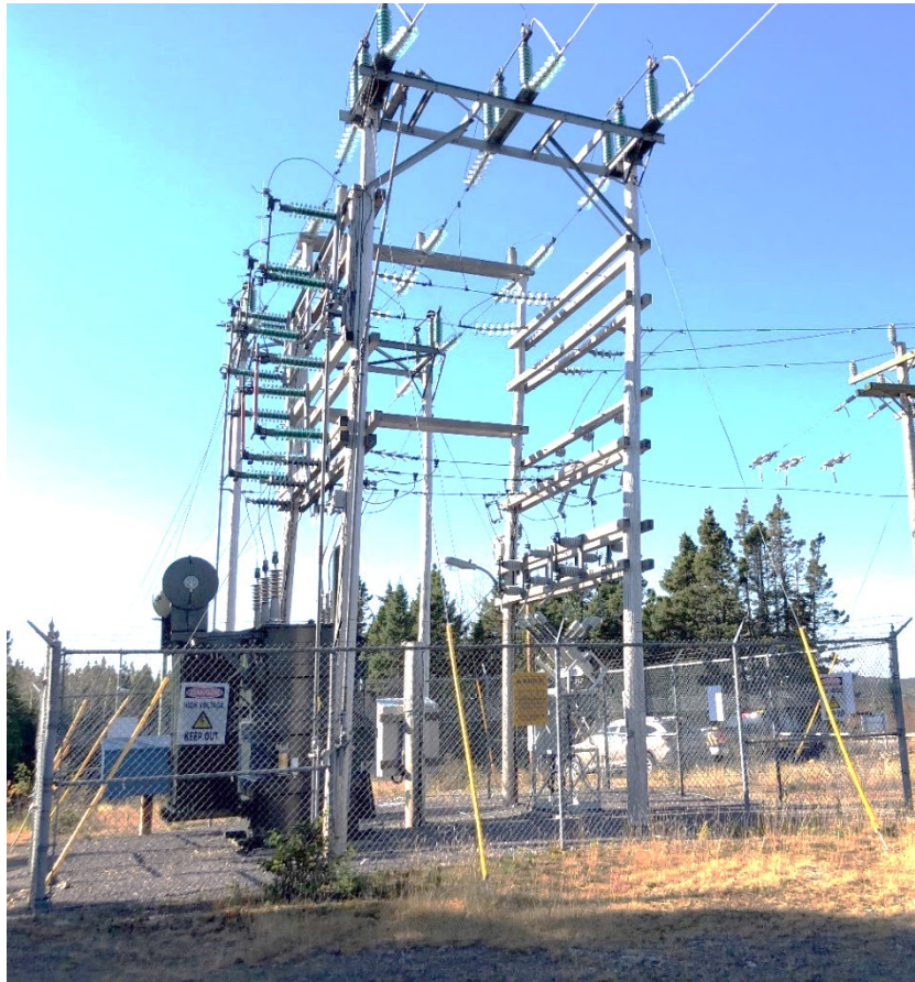
Figure A-1: SMV Substation
