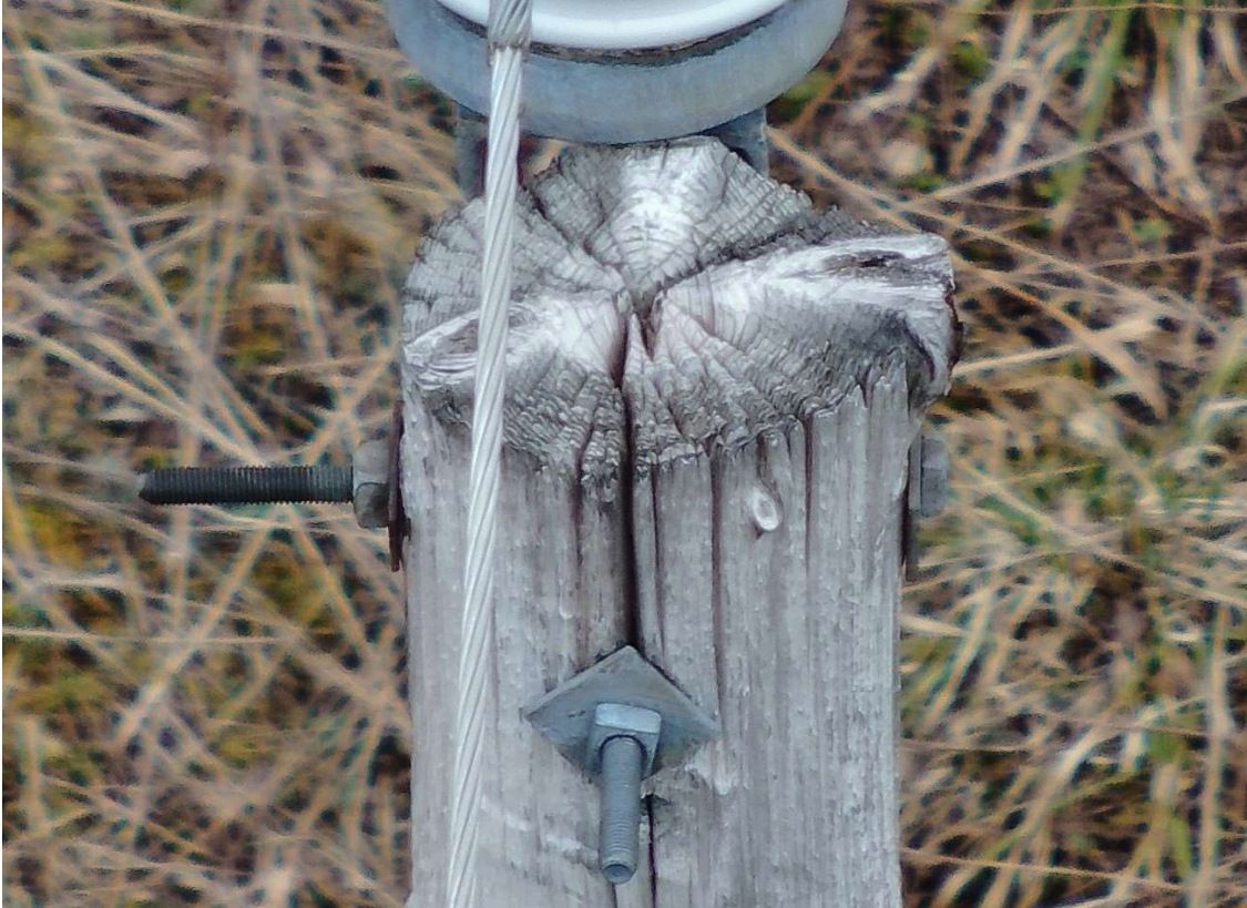
Figure A-6: Pole Top Splits Through Hardware; Narrowing of Pole Top
