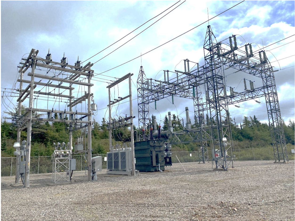
Figure B-1: NWB Substation
