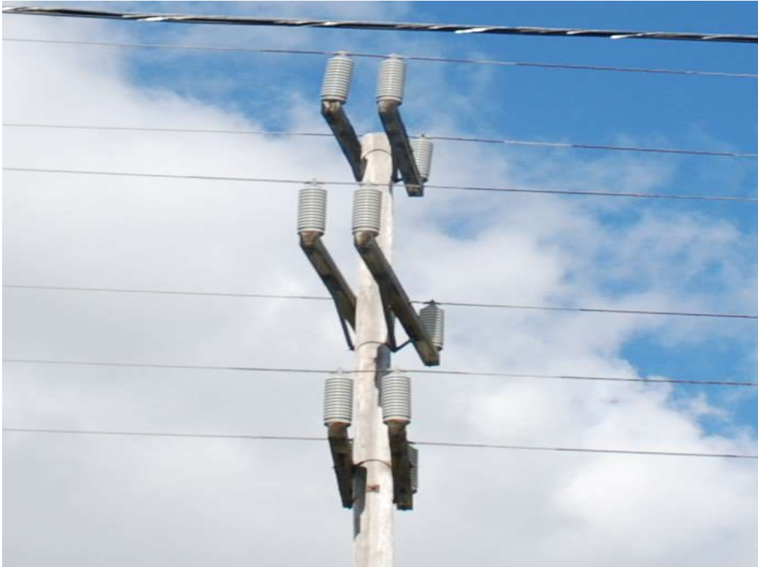
Figure A-12: Twisted Cross Arms (Double Circuit Structure)
