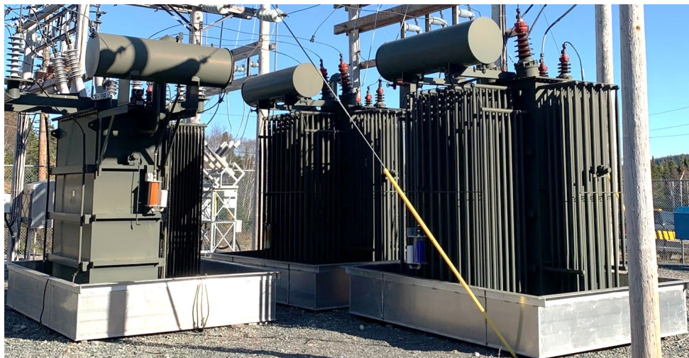
Figure C-7: LOK Hydro Plant Transformers (LOK-T1, LOK-T2 and LOK-T4)
