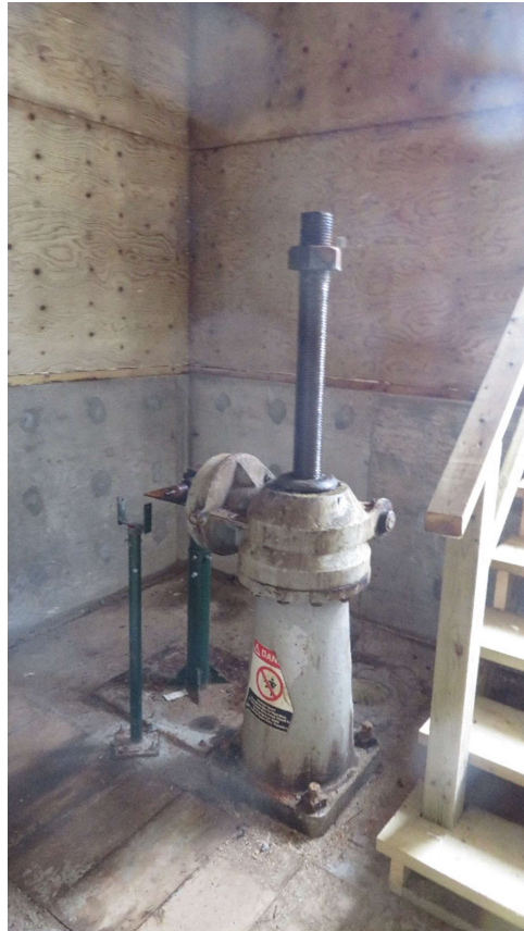
Figure 10 – Outlet Gate Operator
