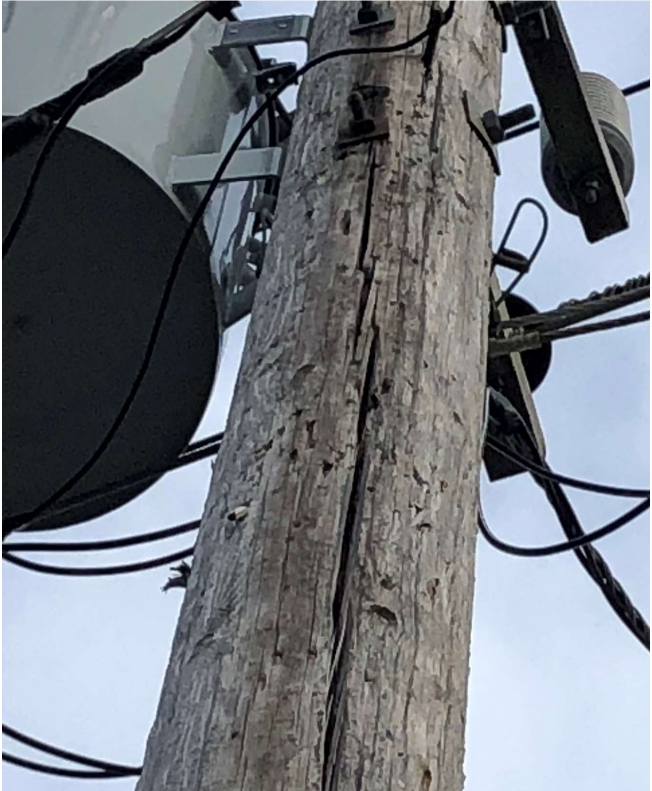
Figure A-5: Large Split, Hollow Pole (Shared Transmission/Distribution Structure)
