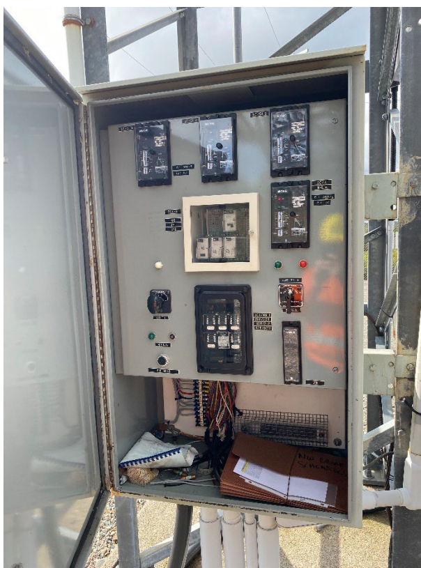
Figure B-5 - 138 kV Bus, NWB-T1 Protection Panel
