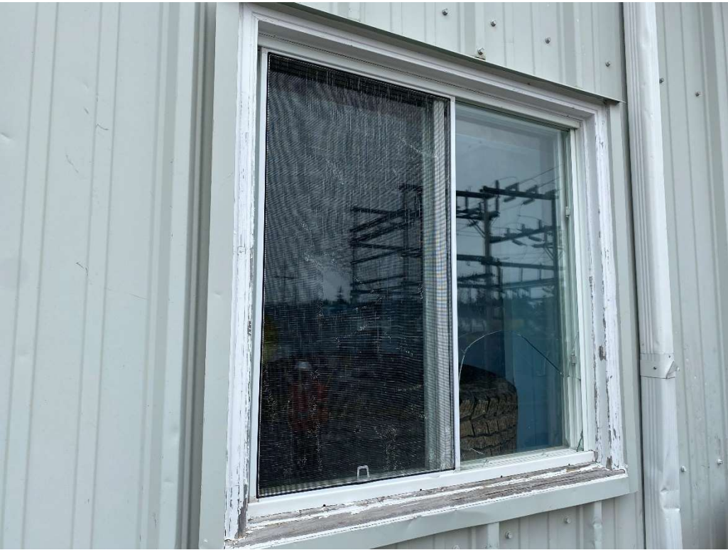
Figure 3: Exterior Window Deterioration
