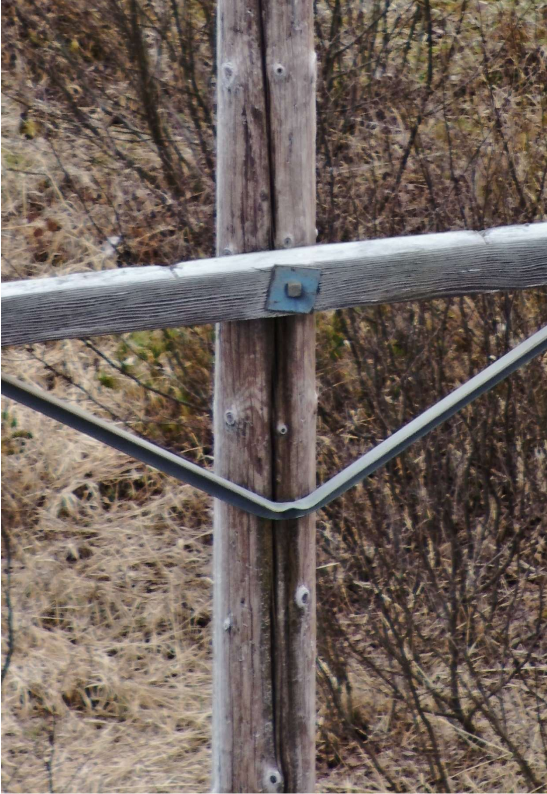
Figure A-4: Large Split Through Cross-arm Hardware
