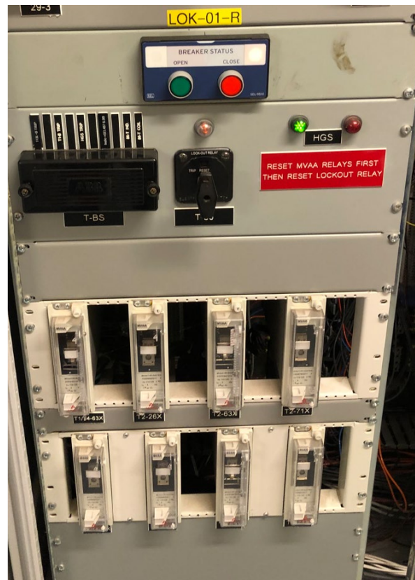
Figure C-8: LOK-T1, LOK-T2, LOK-T3 and LOK-T4 Protection Panel
