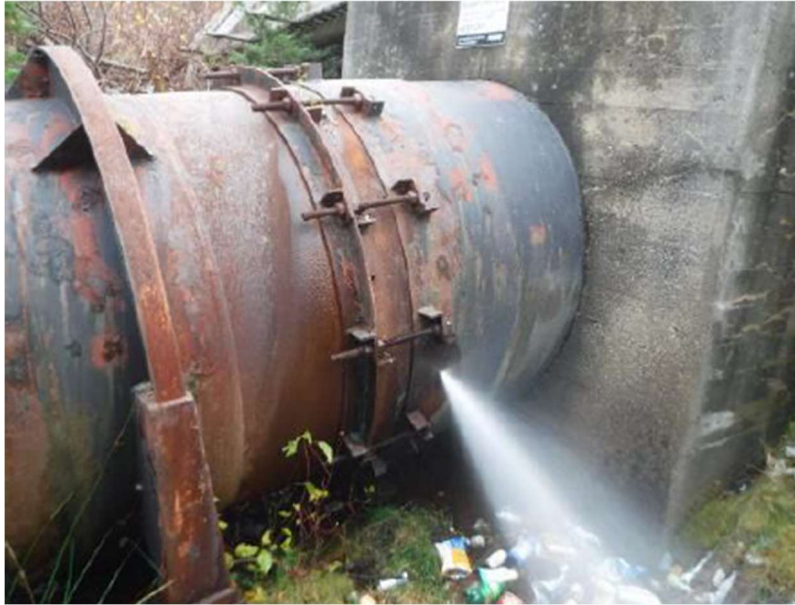
Figure 2: Expansion Joint Leakage
