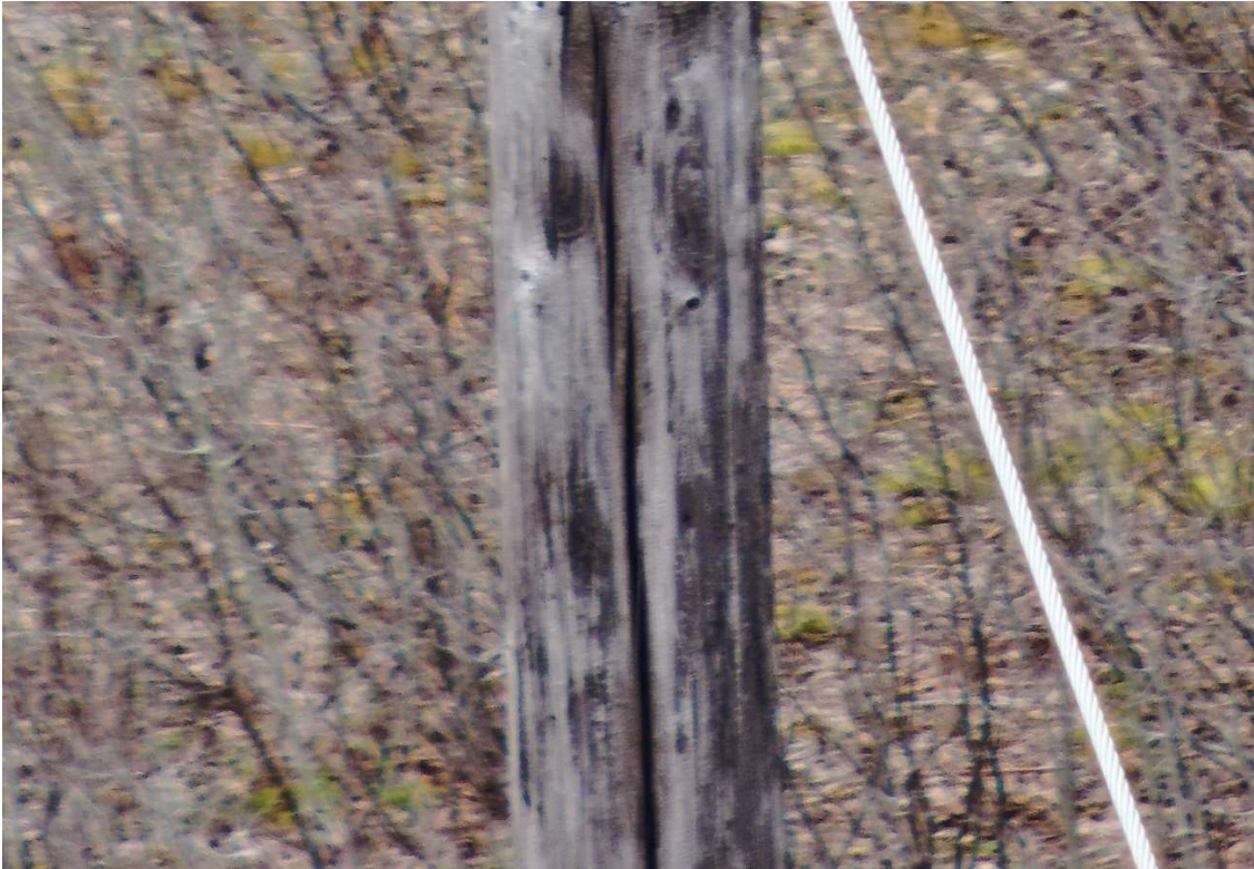
Figure A-7: Deep Splits Through Pole
