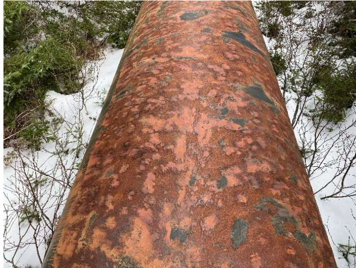
Figure 1: Protective Coating Loss
