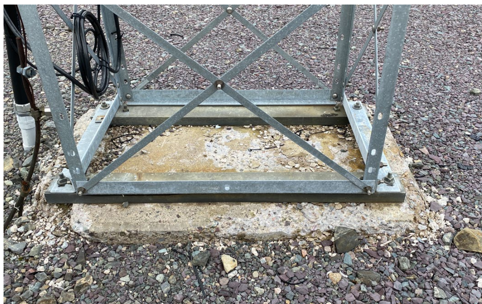
Figure A-5: Recloser Deteriorated Foundation
