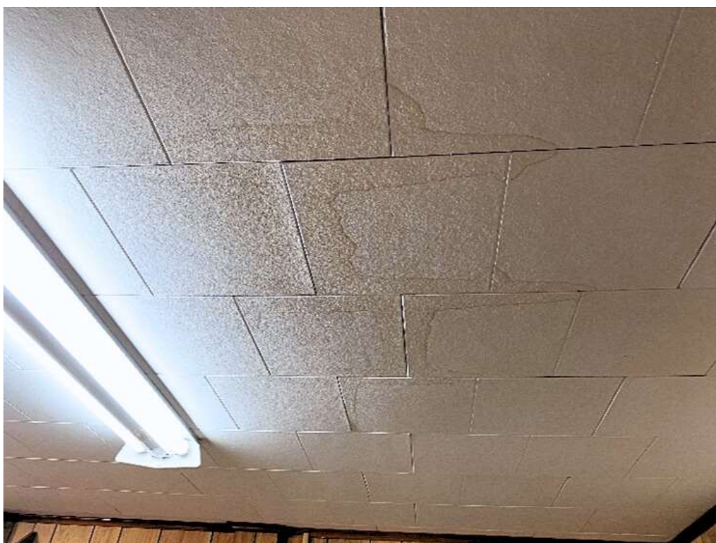
Figure 4: Ceiling Moisture Damage
