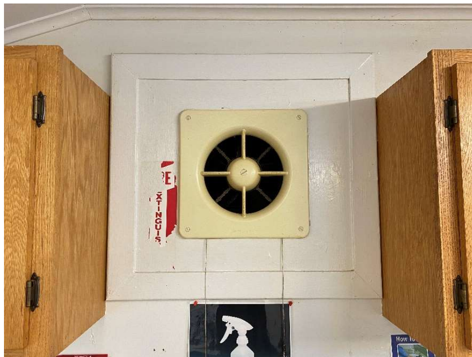
Figure 7: Kitchen Exhaust Fan
