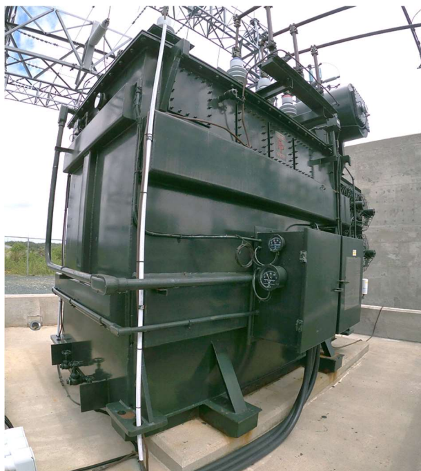
Figure A-2: Power Transformer PUL-T2
