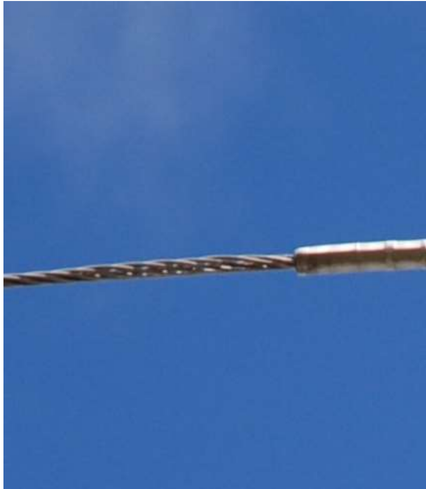
Figure A-13: Conductor bird-caging
