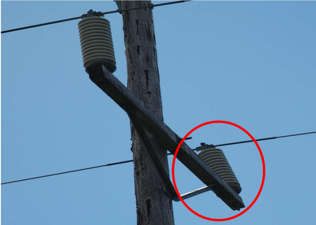
Figure A-11: Twisted Cross Arm Supporting Insulator
