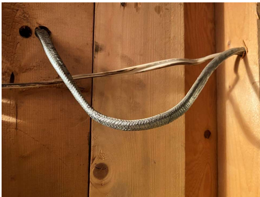
Figure 8: Cloth Insulated Wiring
