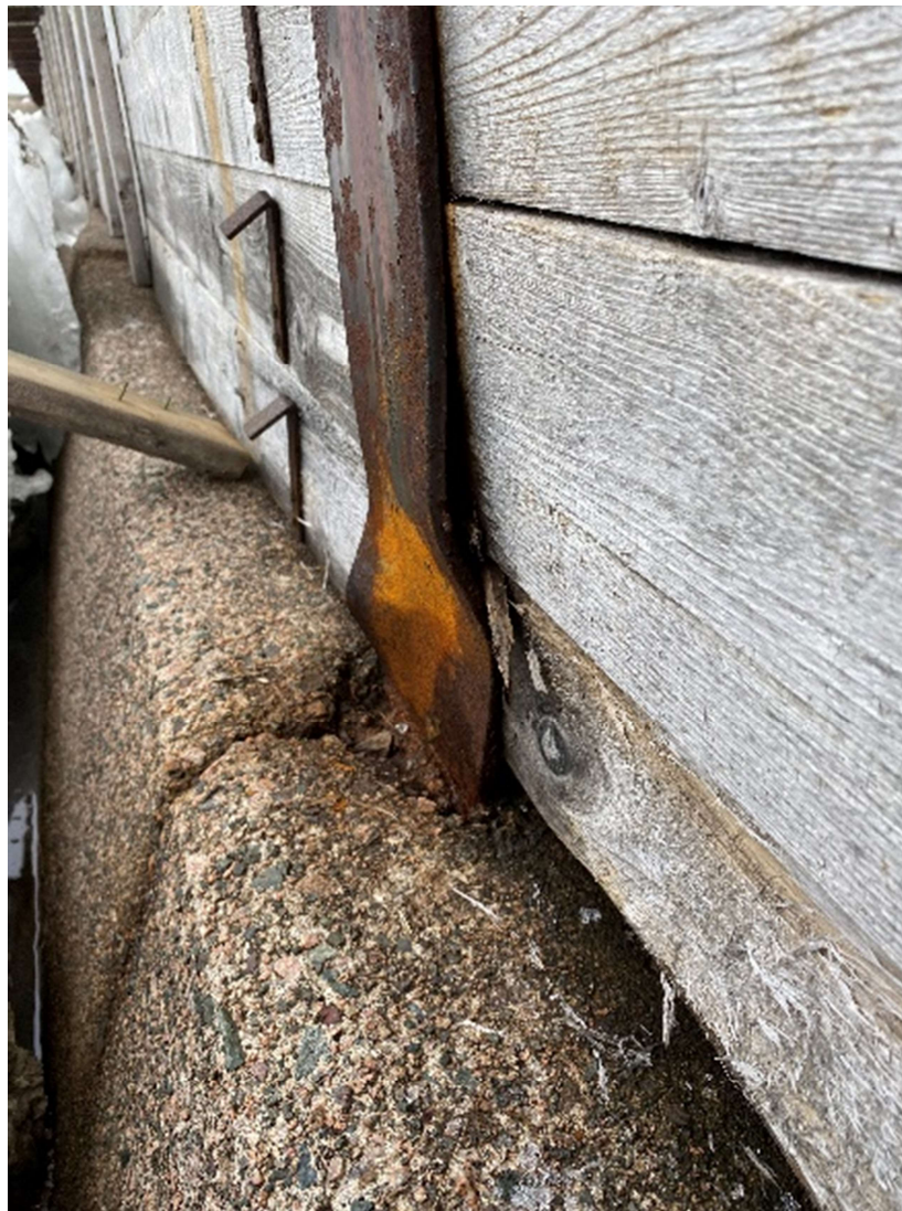
Figure 6 – Damaged Stoplog Support
