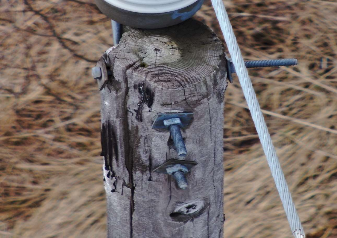
Figure A-8: Deteriorated and Narrowed Pole Top
