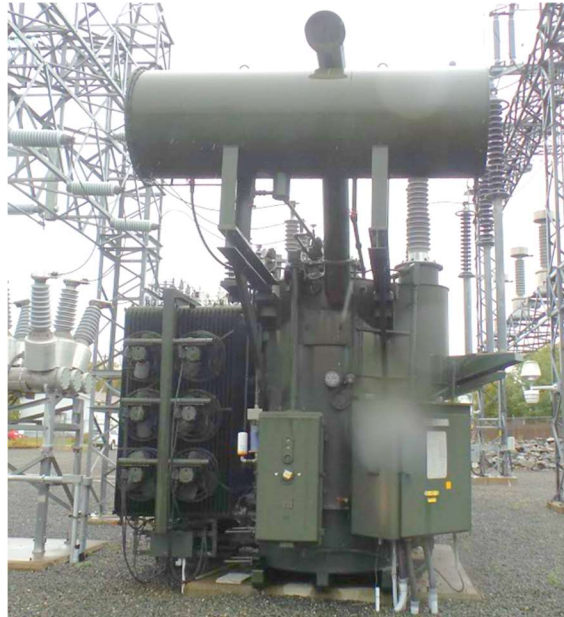
Figure B-3: Power Transformer GAN-T2
